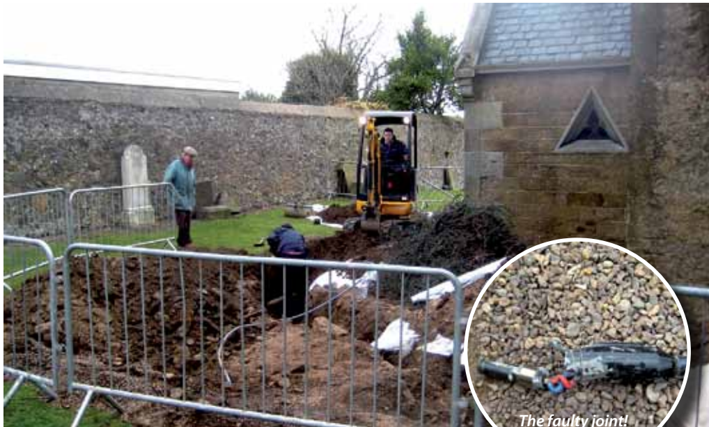
The faulty joint!
